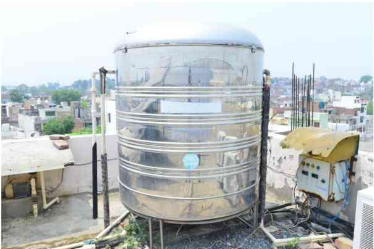
R.O. Water Storage Tank
